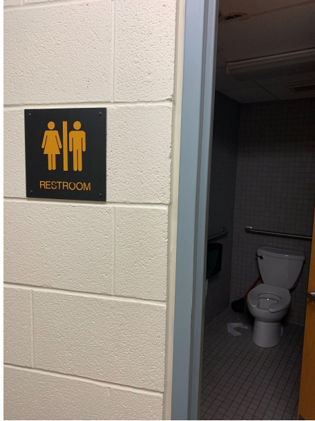
Caption: The Gender Neutral Bathroom in the Whalen Center for Music is located within Ford Hall and would be inaccessible if the hall was closed or in use. The signage is not proper.
